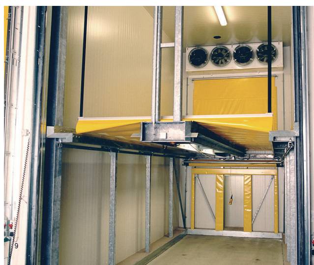
Tarp system ripening room
